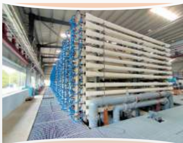
Рис. 3. Ultrafiltration and Reverse Osmosis system for a water recycling plant built by WABAG
